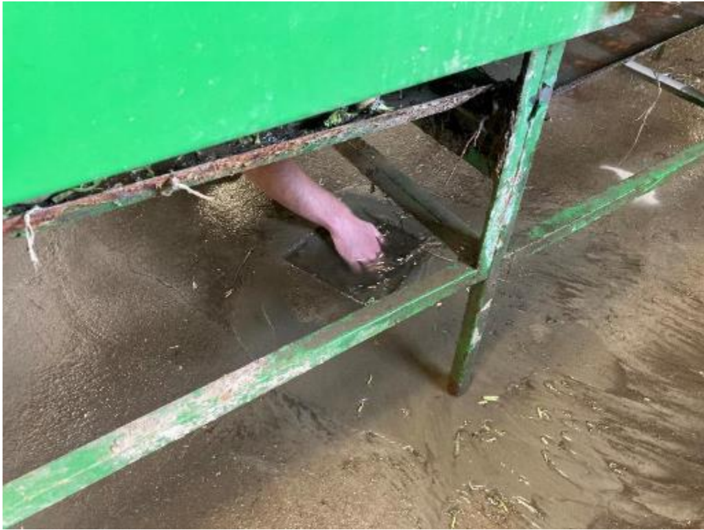
Example of a clogged and overflowing drain
