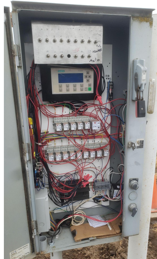
Customer build – Siemens HMI & smart relay — Abandoned PLC for manual switching
